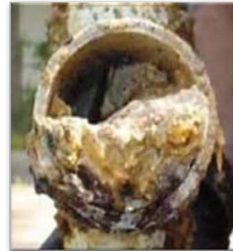
Clogged Sewer Line Caused by FOG
