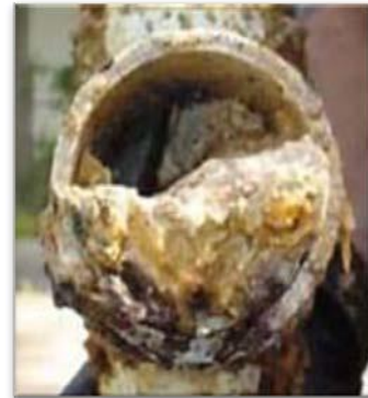
Clogged Sewer Line Caused by FOG
