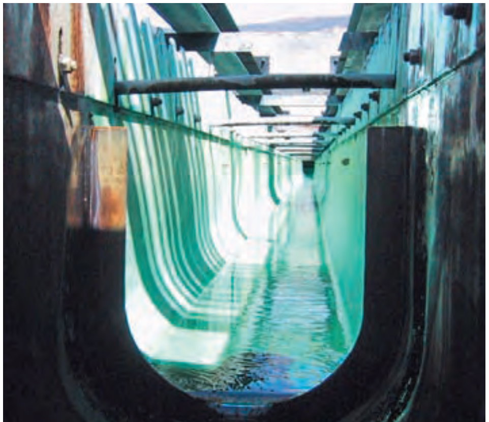
Water flowing in one of the many treatment stages at the Cater Water Treatment Plant.
