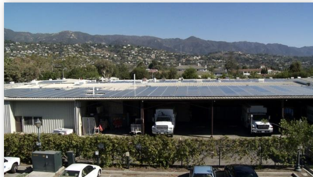
CITY CORPORATE YARD SOLAR PANELS
