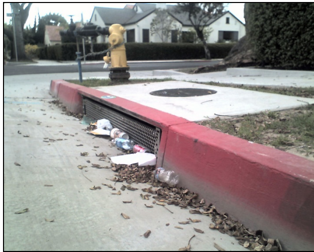
Before – Trash is held at the curb by the screen.
