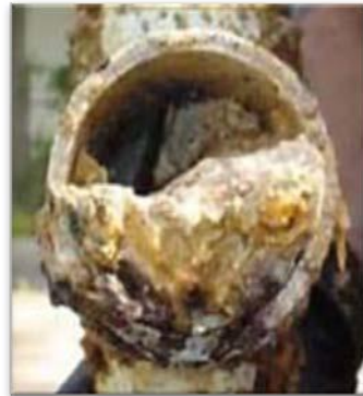
Clogged Sewer Line Caused by FOG
