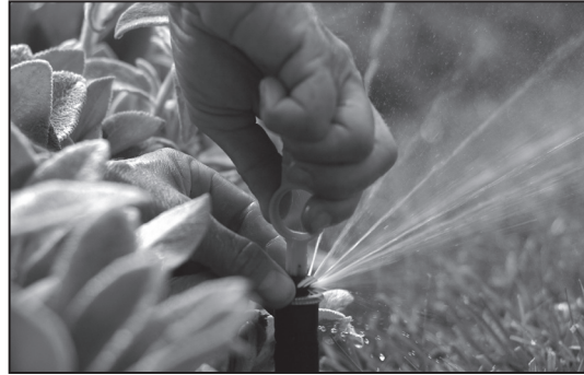
Use the Irrigation Startup Checklist to prepare your irrigation system for summer.
