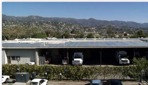
CITY CORPORATE YARD SOLAR PANELS
