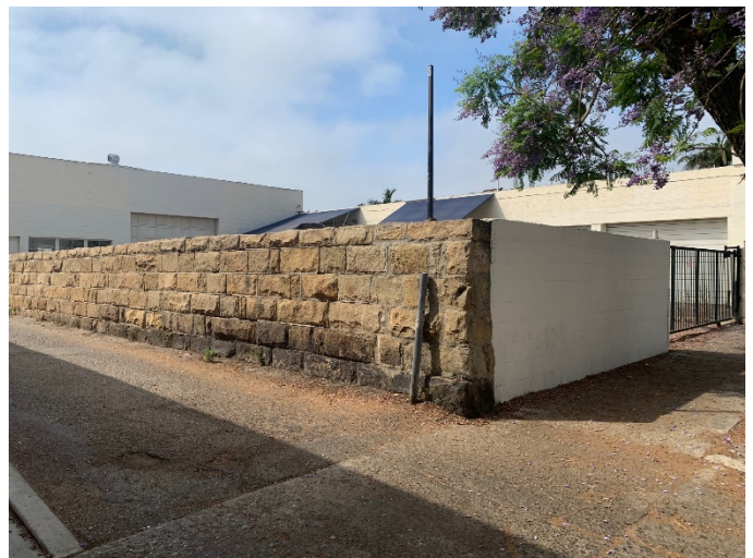
View of six course, ashlar cut wall from West Ortega Street facing west.
