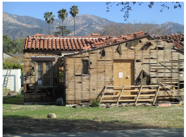
Photograph of house after exterior work started without permits.
