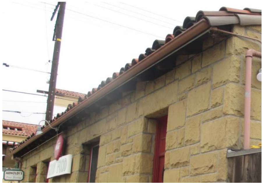
Above: The restaurant was constructed with high-quality materials, including terra-cotta roof tiles; simple, rounded, wood brackets under the eaves; and ashlar cut sandstone walls. Photo taken February 2, 2016.
