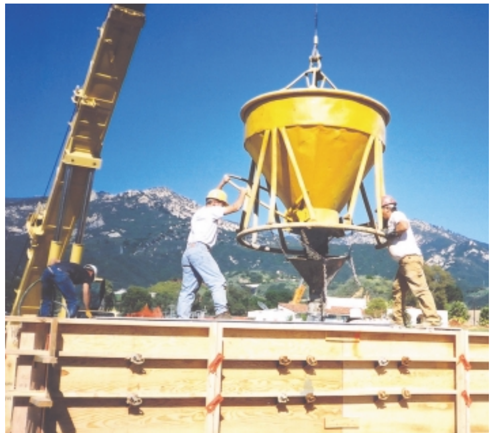
Crews pouring the concrete walls for a new pump station at the William B. Cater Water Treatment Plant.
