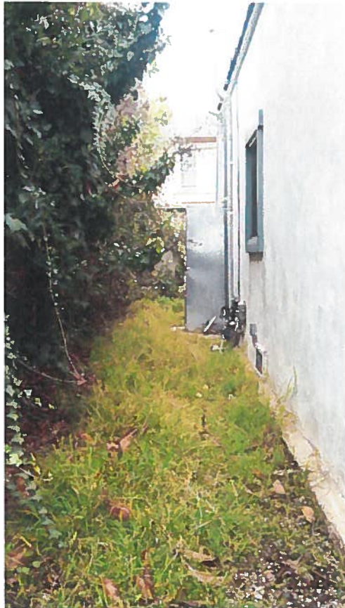
"As-built" water heater enclosure
