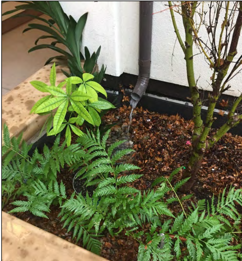
FIGURE 5-3: Downspout Directed to Landscaping in Santa Barbara
